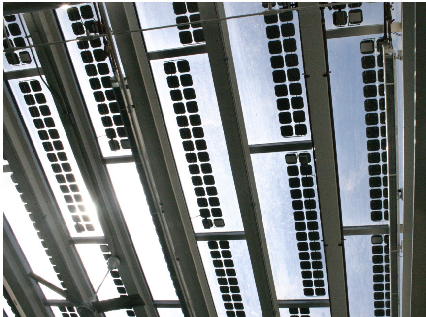
An integrated solar PV system installed in the skylights at the Marjorie McNeely Conservatory at Como Park in St. Paul
